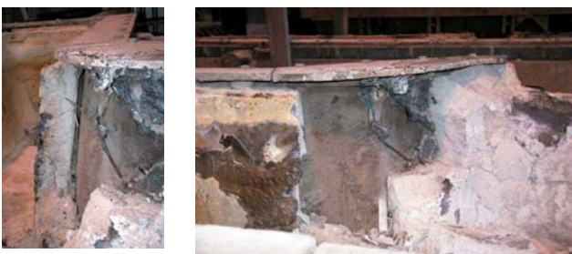
Fig.2: Failure of the safety lining of a T-shaped tundish
