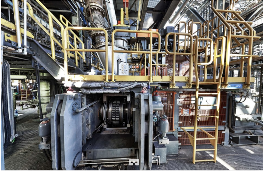
Figure 33: Briquetting deck at voestalpine Texas LLC [51]
