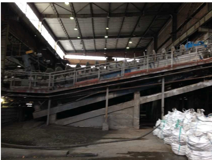
Figure 21 Crushing and Separators, Tunel I pari Process Plant
