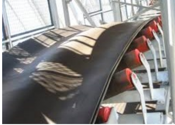
Figure 2-21: Belt deformations caused by the bulk material in a sandwich conveyor (Snake Conveyor by DSI) [60]
