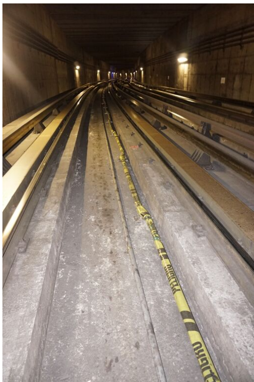
Fig. 3.21 Photograph of the inclinometer rods (covered with the yellow tape) mounted in a tunnel along the track, © Geodata GmbH.
