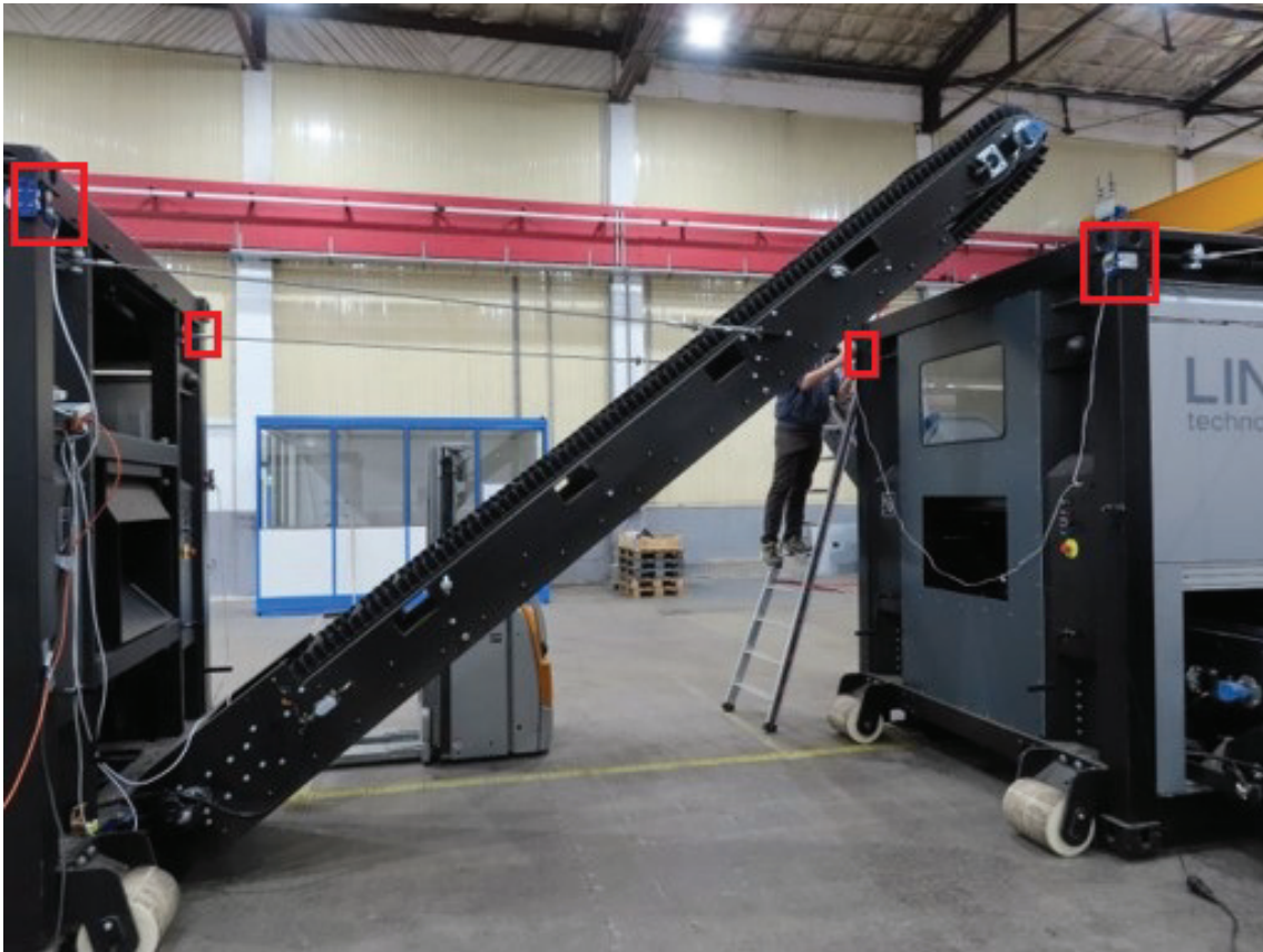
Figure 6.9: Second constellation of field tests: For the final system verification the developed system is installed on plant units in an assembly hall, now connected through conveyor belts. The sensors are mounted at the top of each edge - marked by red rectangles - and connected to the power supply. Only the Anchors are additionally connected through Modbus RTU to the IPC as well.
