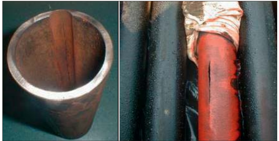
Fig. 4 Typical tubing failure
