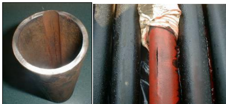
Figure 4: Typical tubing failure
