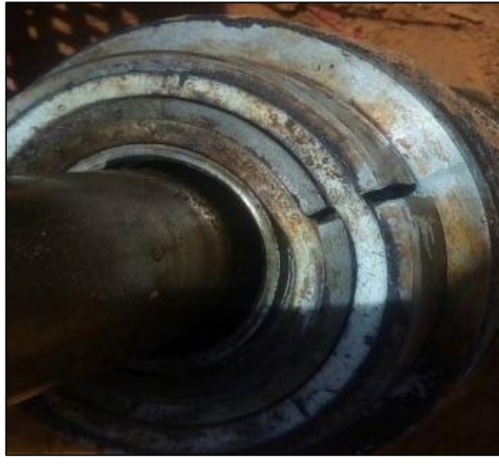
Figure 23: Stuffing box split due to misalignment issue.
