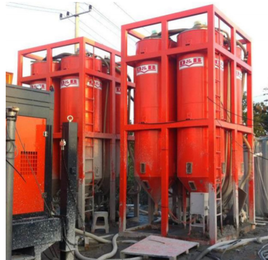
Figure 42: Cutout of the sedimentation and lamella cleaning system used by Hanjin 2
