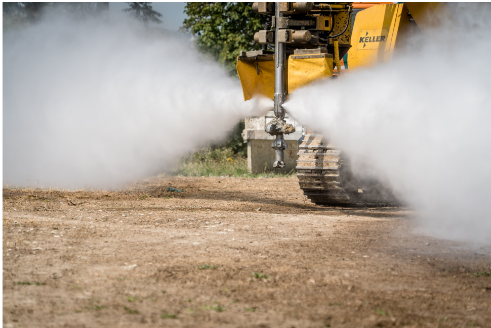
Figure 2.28: Jet Grouting Drill Bit with Jet Nozzles ( Courtesy of Keller ): The figure shows the location of the jet nozzles on the monitor at the bottom end of a drill string. Water exits the nozzles at high pressure. This is only one out of many different configurations of jet nozzle size, number and spatial distribution, as described in Figure 2.27.
