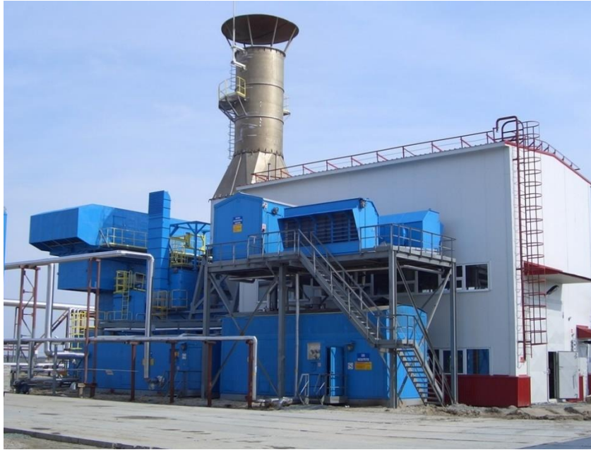
Figure 7 - Compressor unit at compressor station №7
