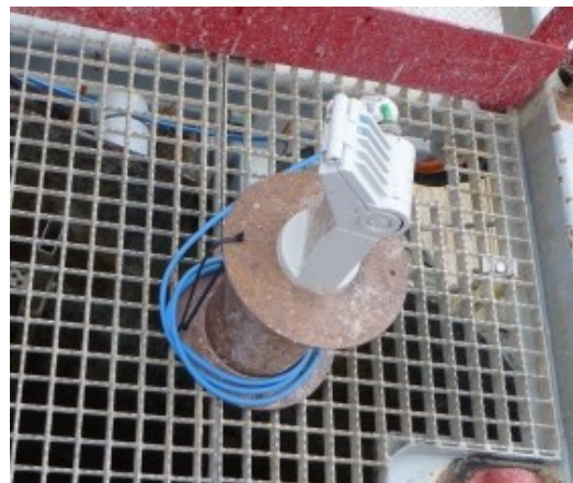
Figure 10: Most common pit level sensor positioning, without any protection against incorrect measurement due to foam.
