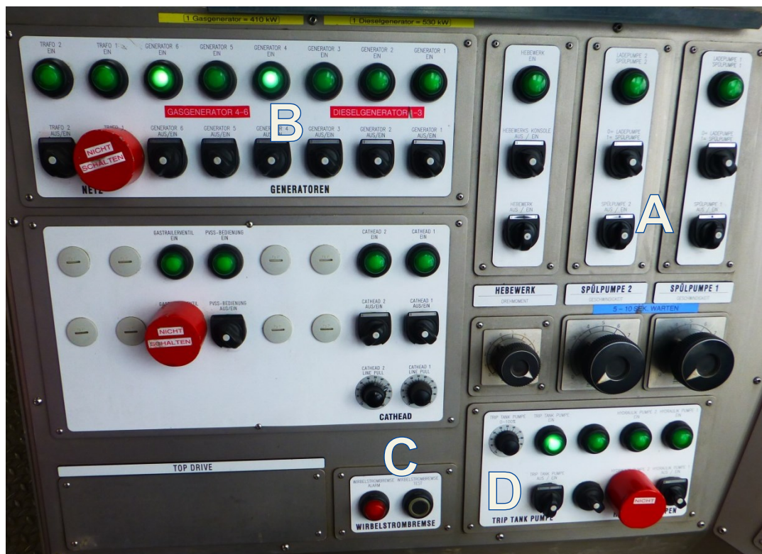
Figure 7: Main control panel located to the left of the drillers view on the drillers console
