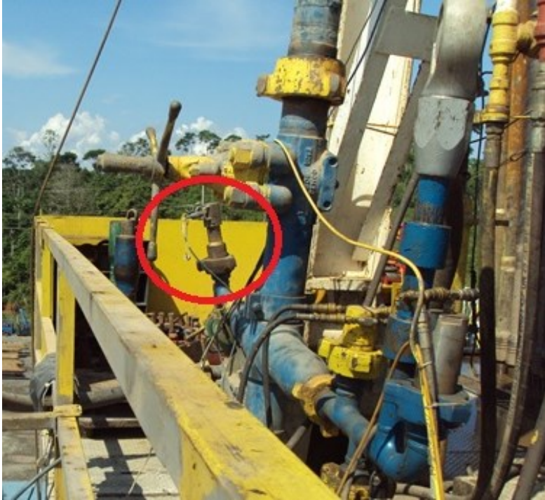
Figure 9 Pressure Transducer installed in manifold on the rig floor
