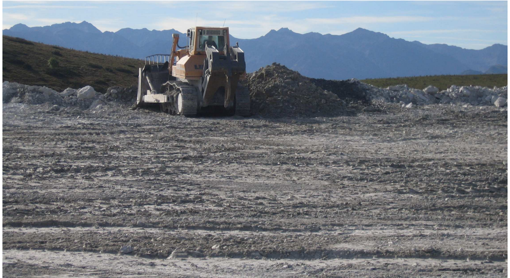
Figure 6.16: Bad road conditions at dump site
