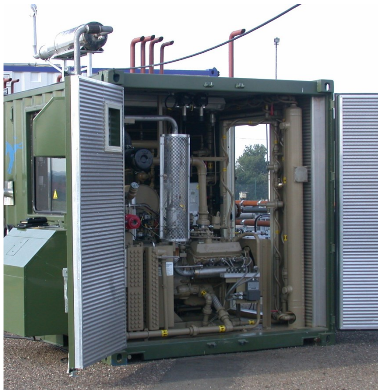
Figure 36: GasJack housed by offshore container
