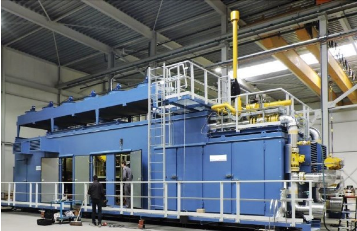
Figure 33: Screw compressor, which is installed in a container
