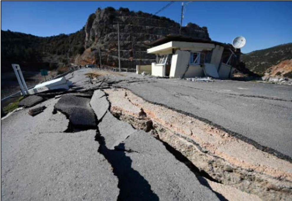
Figure 16: Destroyed road in Turkey. Source: thenationalnews.com
