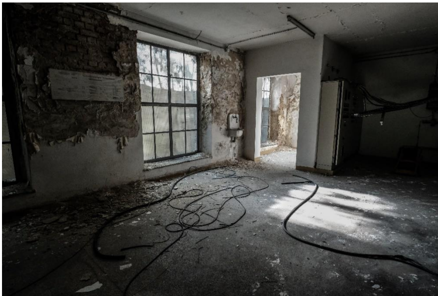
Figure 47: Damage to ceiling and walls due to moisture ingress
