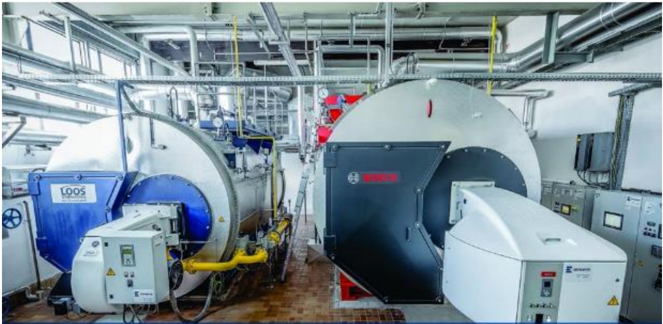
Figure 27: Boiler plants for process steam generation [Picture: Edtmayer]
