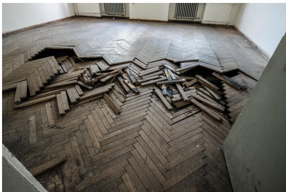
Figure 49: Damage to parquet flooring
