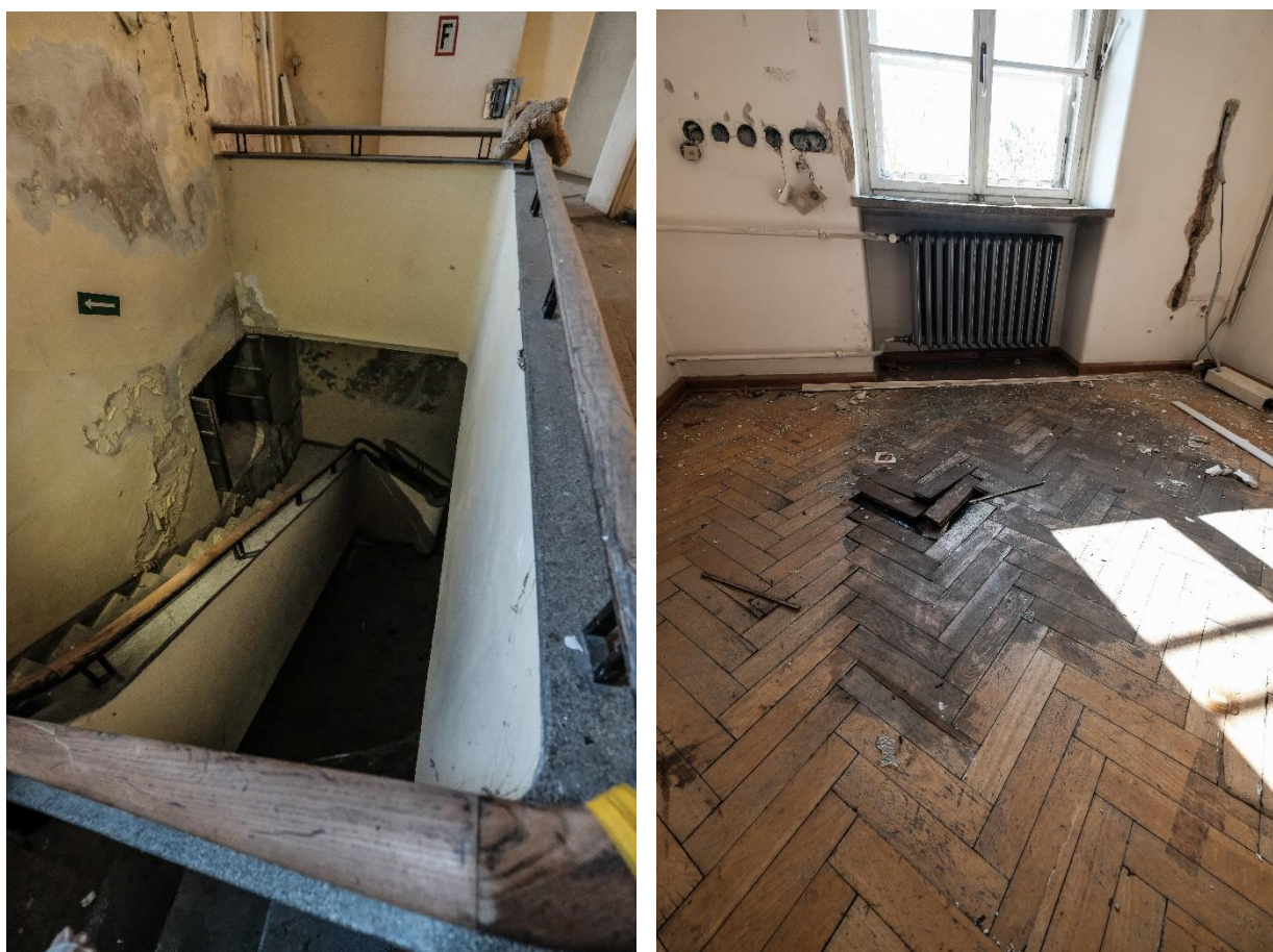
Figure 46: Damage patterns in different indoor spaces.
