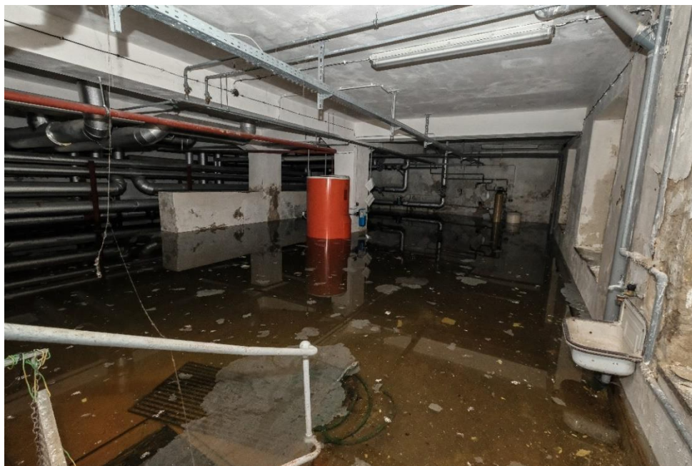
Figure 48: Cellar room with considerable water ingress
