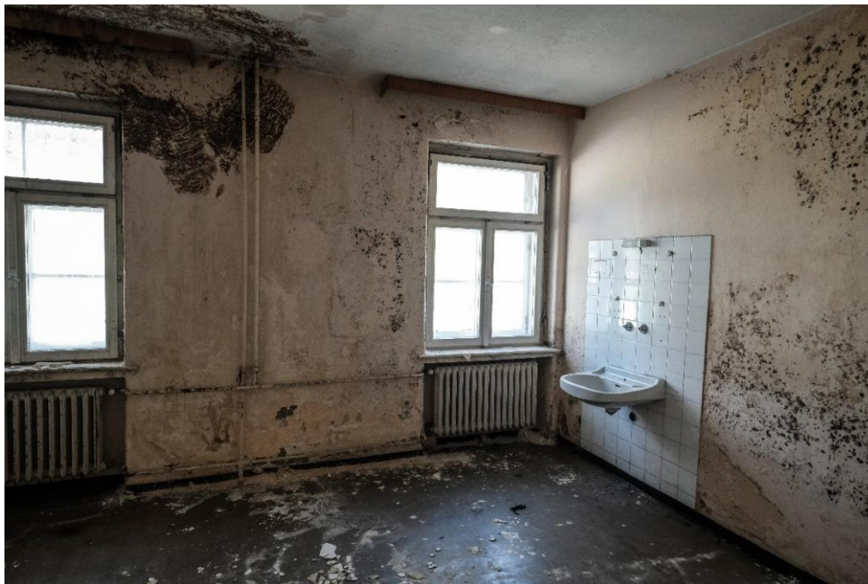
Figure 50: Interior with considerable moisture damage.
