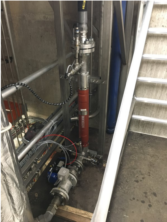
Figure 66: REDA D2400N installed in the facility
