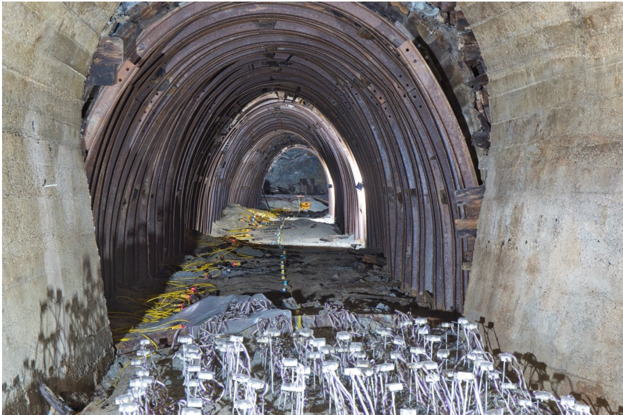
Figure 3: Image showing the starting point of the steel arch section up to the tunnel face. The 101 steel arches give the tunnel its name. In the foreground are the measurement boxes of the 3D ERT visible. A measuring tape can be seen along the profile and the geophones on the left side of it.
