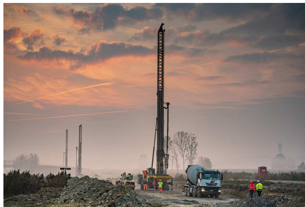
Figure 2: Here a series of three instrumented rigs can be seen on a building site. This gives an impression of the scale of operations and the relevance of location registered data.
