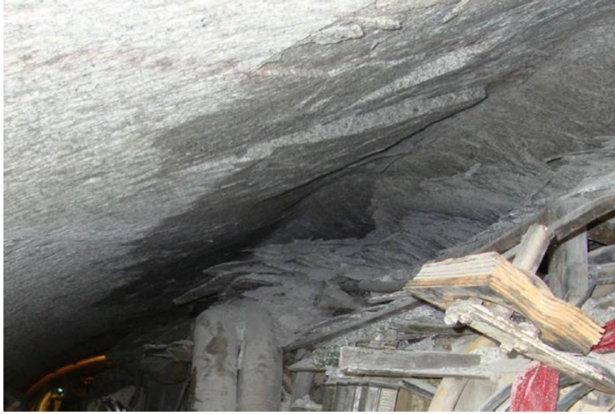
Figure 2.3: Progressive rock spalling above a TBM excavating in granite [13]
