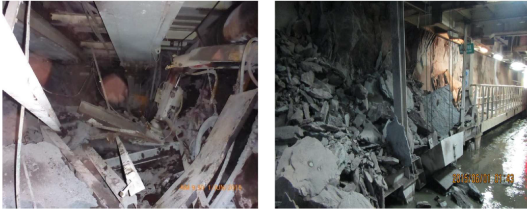
Figure 4.60: The damages caused by the rockburst on the May 31, 2015 in Neelum Jhelum project [111]
