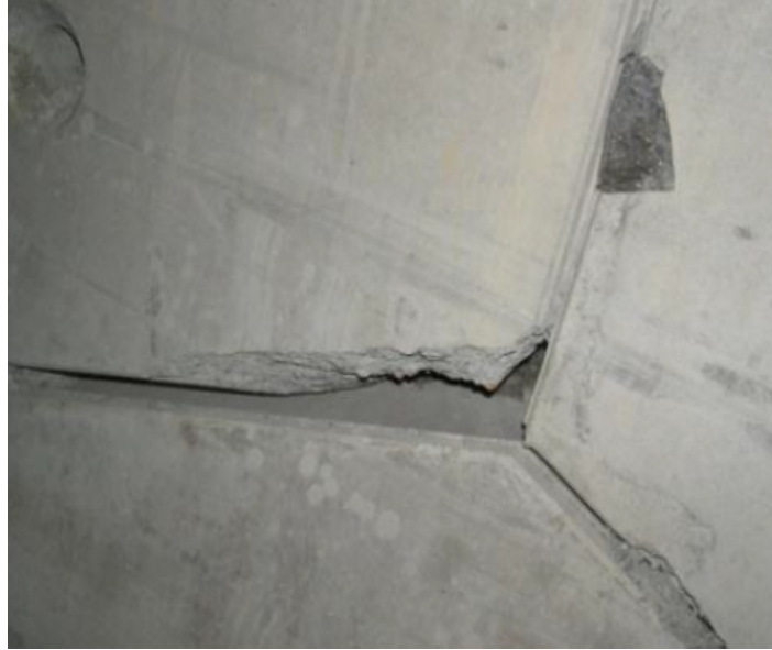
Figure 4.21: One example of the damages to the segments taken place before the installation of the segmental lining
