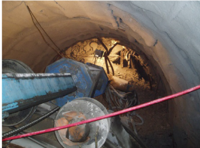
Figure 2.13: An extremely intense rockburst in the drainage tunnel of Jinping II hydropower Station project leading to the total destruction of the TBM [18]
