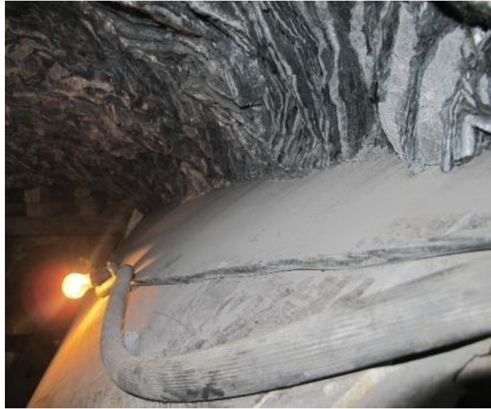
Figure 3.2: The jammed shield of the double-shielded TBM in Golab tunnel [6]
