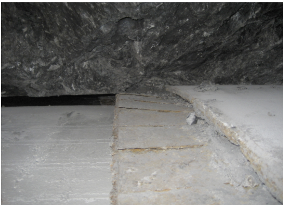
Figure 3.12: The jamming of the shield in Uluabat tunnel [90].
