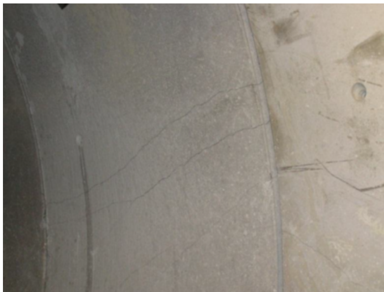
Figure 4.22: Shear cracks in proximity to the adjacent segment junction
