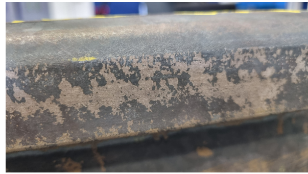
(b) The rail head's surface on the outside of the rail was mostly in a slightly corroded state.
