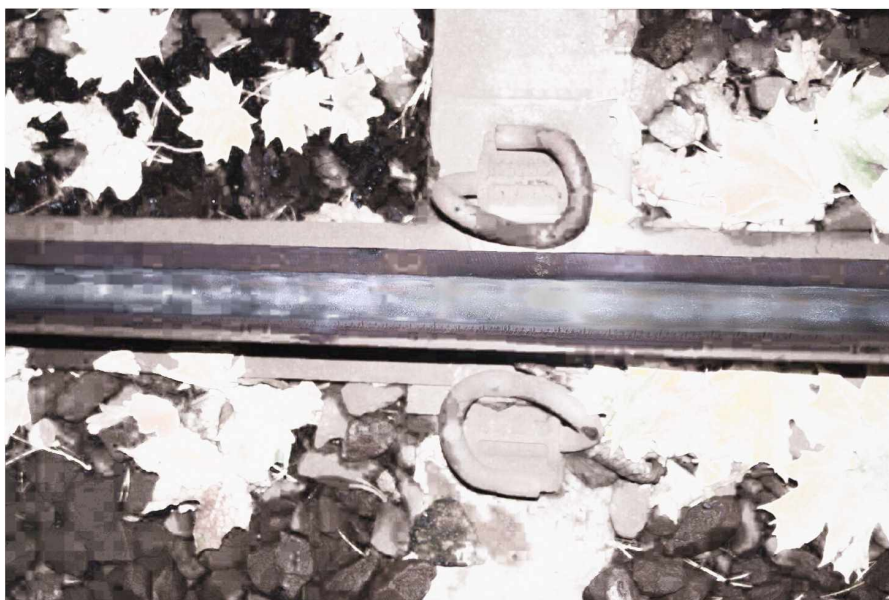
Figure 5.5.: Corrugation on a low rail in a curve, metro system in Scandinavia. Picture provided by P. Torstensson from CHARMEC.
