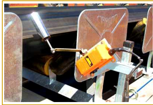
Figure 6-3: Misalignment (off-track) switch on site.
