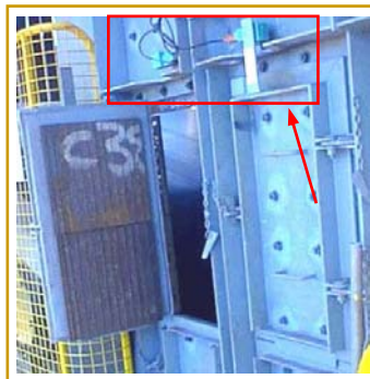
Figure 7-17: Chute access door closed proximity switch.
