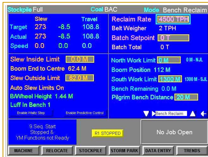
Figure 7-3: Stacker/reclaimer control panel.
