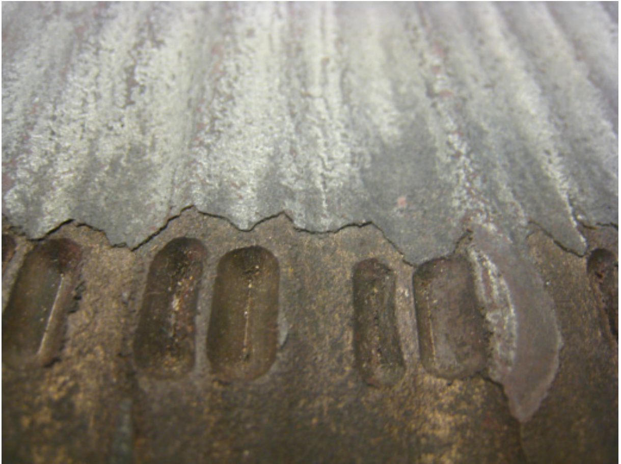
Figure 7.2.: Detail of Figure 7.1: transition between oxide scale and base material. The scale appears glossy, the underlying steel diffuse.
