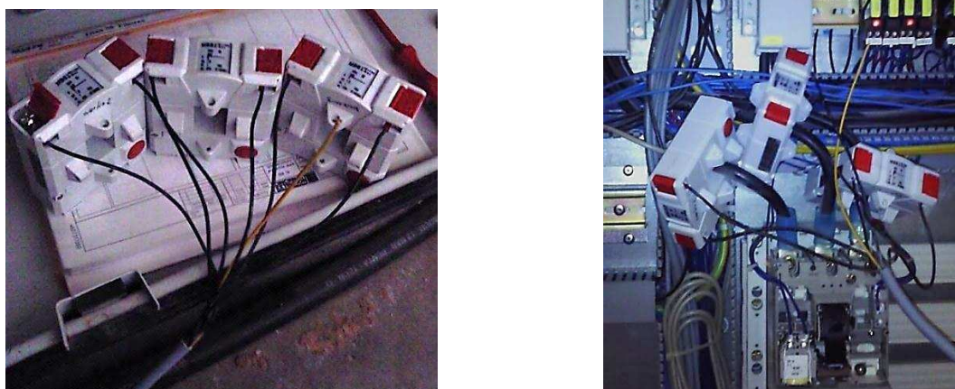
Figure 28: Wired converters – 3-phase cable (left), installed converters flapped over the main supply.
