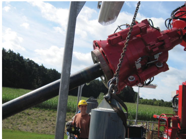
Figure 39: Tilted top drive with CDS while casing is stabbed inside the CDS from the pipe handler on the TBA200
