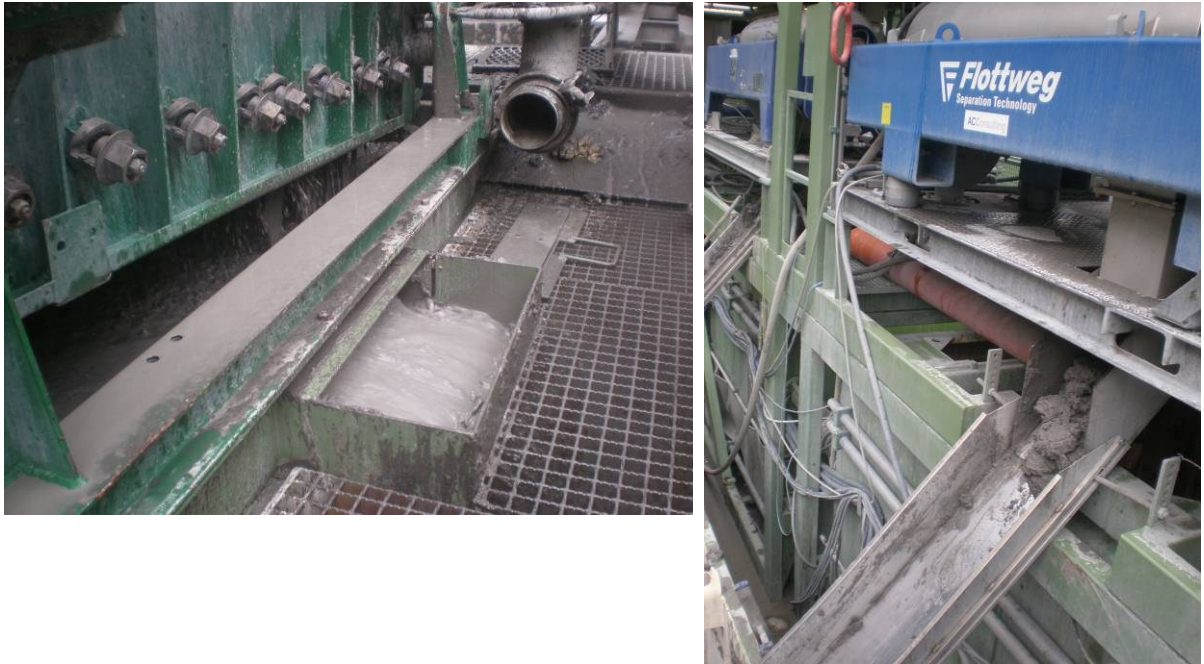
Figure 18: Left Picture - Mud at Screen Underflow of Shale Shakers (Mud Passing the Sieves and Flowing into the Tank); Right Picture – Flocculation Unit Discharge
