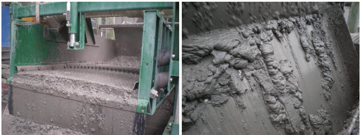
Figure 17: Left Picture - Cuttings Flowing Over the Shale Shakers; Right Picture - Very Fine Cuttings at the Shale Shaker Discharge
