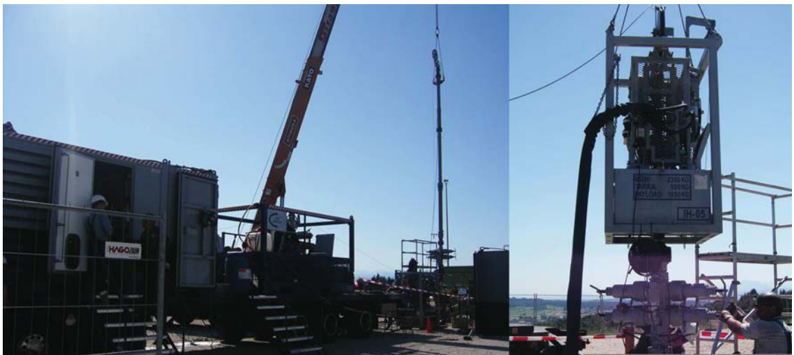
Figure A 12-4 LEFT: Lubricator and BOP for Gauge Run; RIGHT: Injector-Head and BOP
