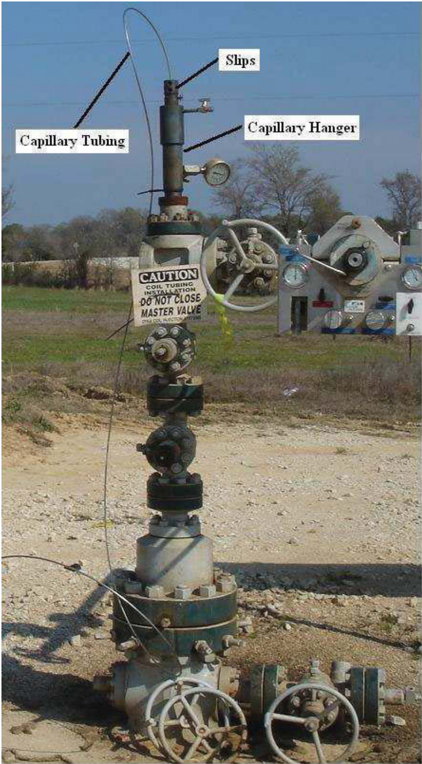
Figure 5-9 Capillary Hanger screwed into the Wellhead Top Flange (a well in the USA) 33
