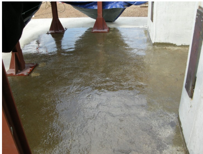
Figure 7: Seal on the floor
