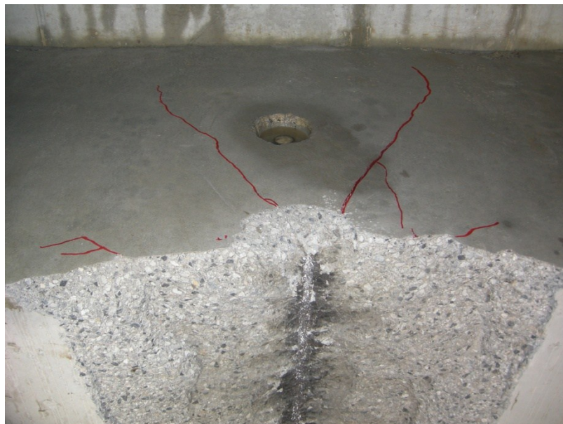
Figure 32: Tracing the blasting cracks
