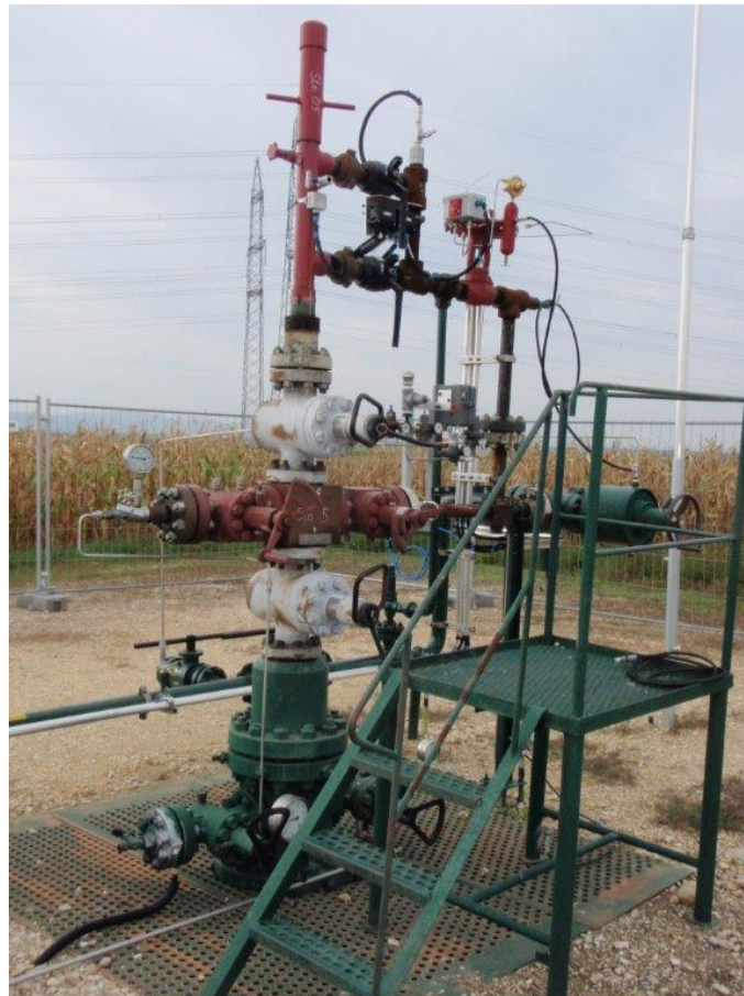
Figure 62: Plunger lift surface equipment - Well 2
