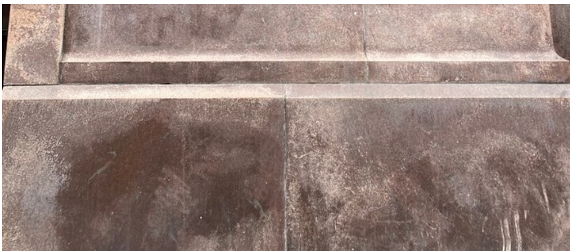
Figure 25. Example of biodegradation on a building facade
