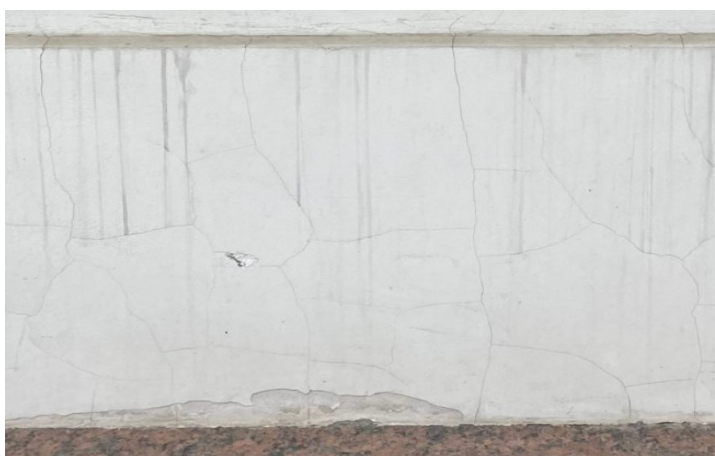
Figure 23: Examples of physical weathering from the facades of buildings in St. Petersburg
