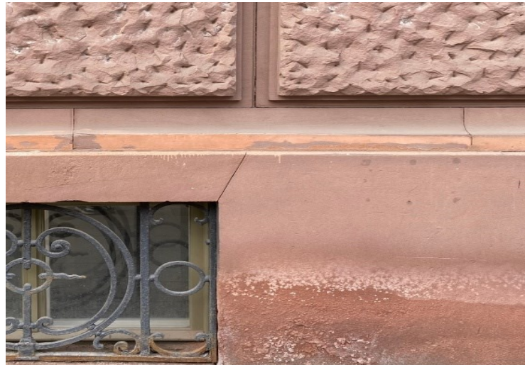
Figure 24. Examples of chemical weathering from the facades of buildings in St. Petersburg
