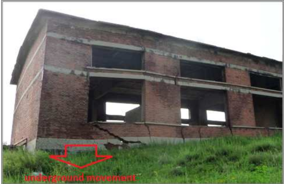
Figure 46: Destroyed buildings indicate underground movement.
