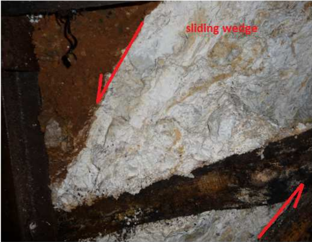
Figure 47: Deep mass movement documented in a closed tunnel in the area of mine 6.
