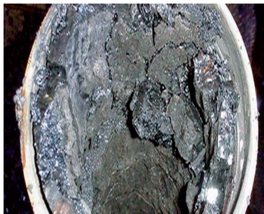
Figure 2.23 – ARPD deposits on the surface of the pipeline
