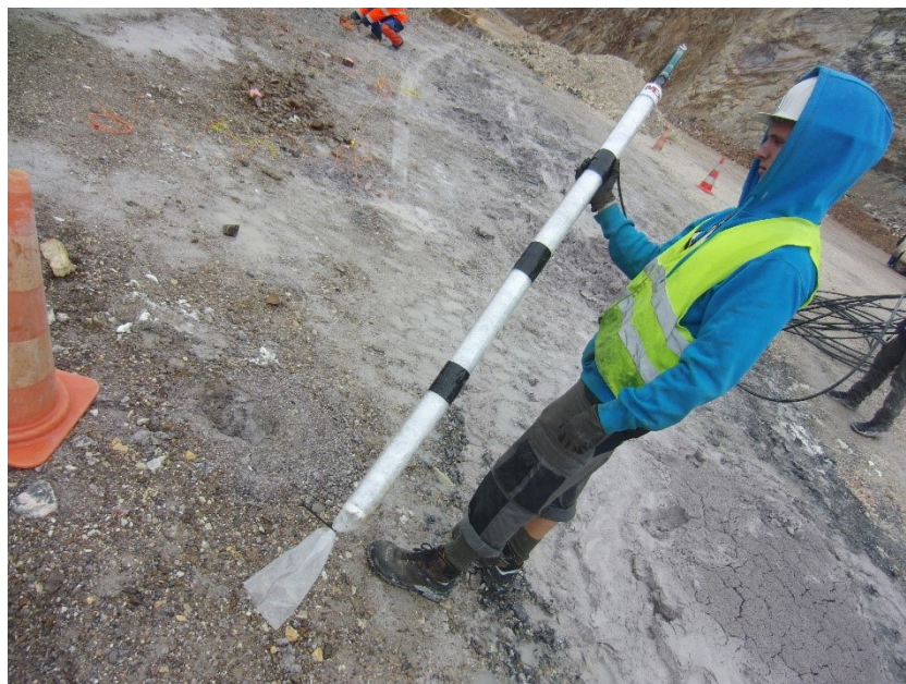
Figure 46: Prototype connected via one-inch tube with a rigid plastic hose, used for high pressured air transportation
