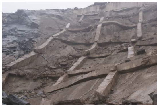
Fig. 1.3 Large Deformation Damage Characteristics of Reinforcement Area on Platform 526m
