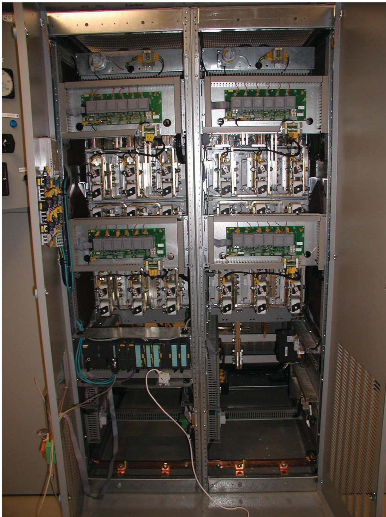
Control System Inside (Phoenix, U.S.A.)
