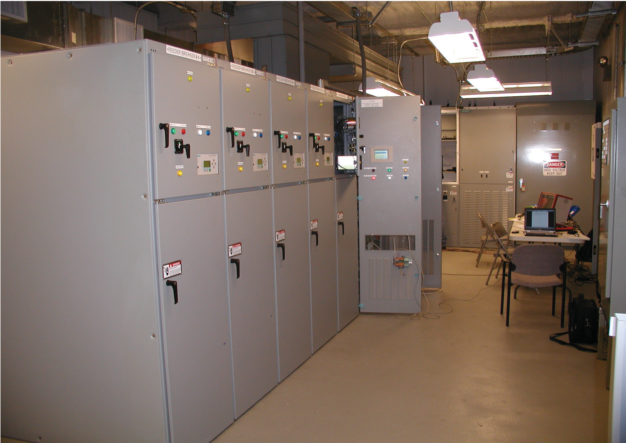
The Substation Control System in Phoenix (U.S.A.)
