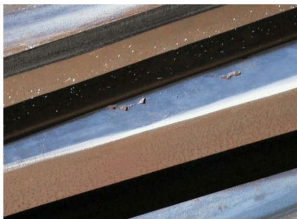
Figure 2: A damaged crossing nose with surface cracks and breakouts.
