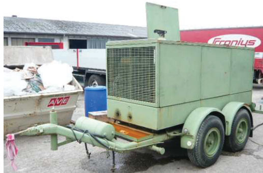
Figure 30: Diesel driven generator with 400 V, 81 A and 50 Hz.
