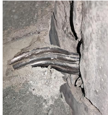
(b) Bending damage of cables
