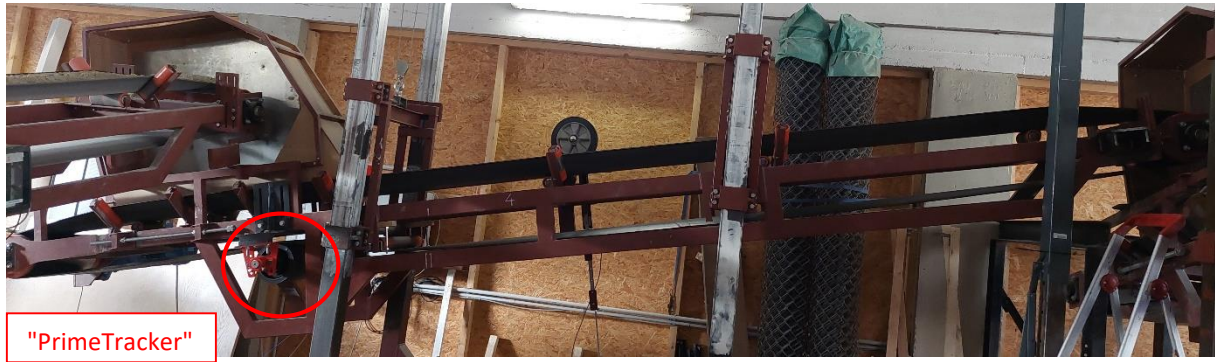
Figure 2 Conveyor circuit with the PrimeTracker installed in one of the four belt conveyors
