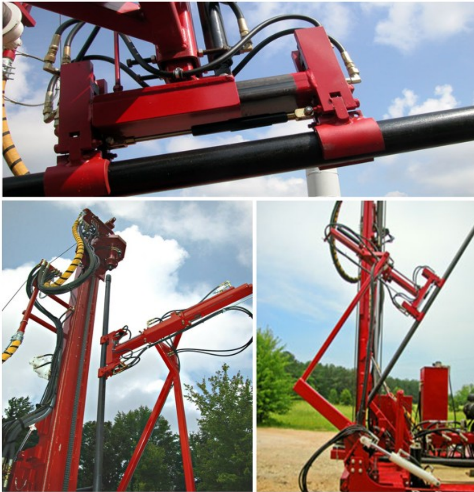
Figure 61: The pipes are clamped and centred onto the top drives axis in order to make the connection, normally performed by the integrated single direction tong of the top drive.
