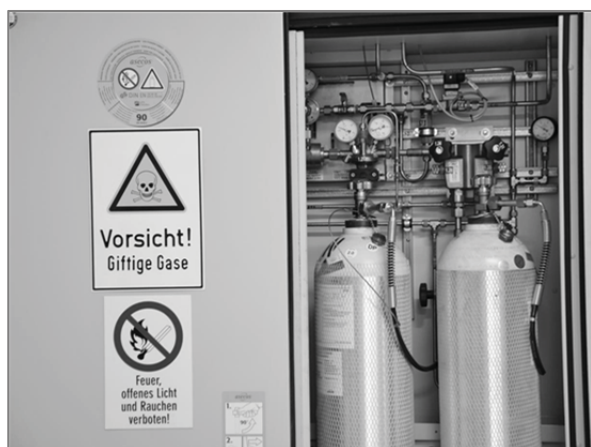
Figure 42: Gas supply unit
