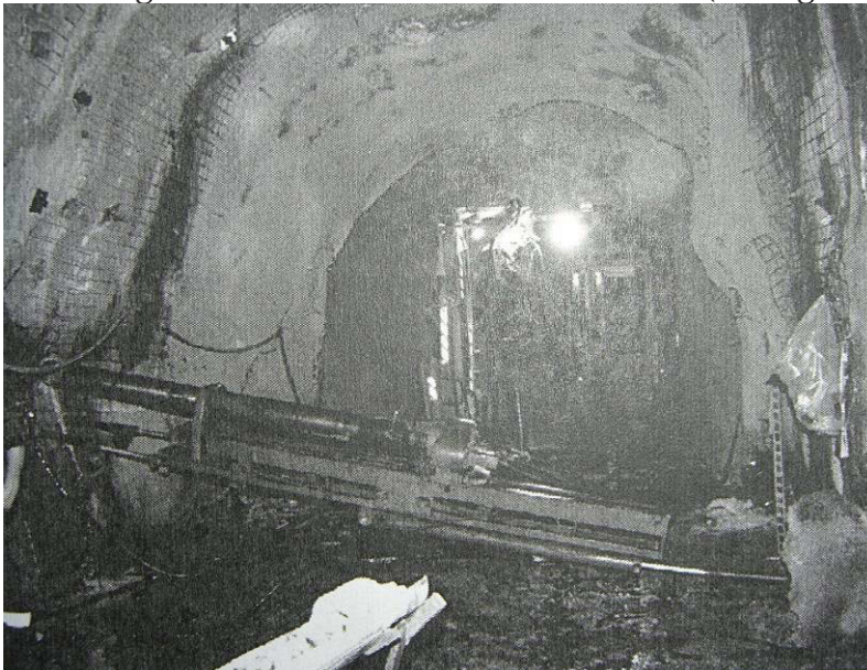
Figure 3-47 WASM bolting overcoring facility (Villaescusa, Varden and Hassell, 2008)
