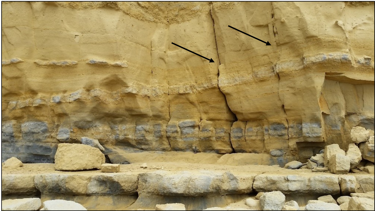
Figure 14: The black arrows indicate the natural fractures
