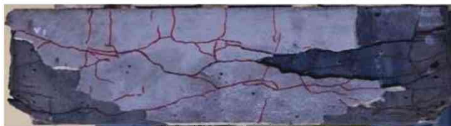
Figure 24: Surface cracks detection. Back side block CH01B04
