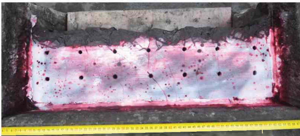
Figure 35: Crack detection at the top of block after 1st row blast block B09
