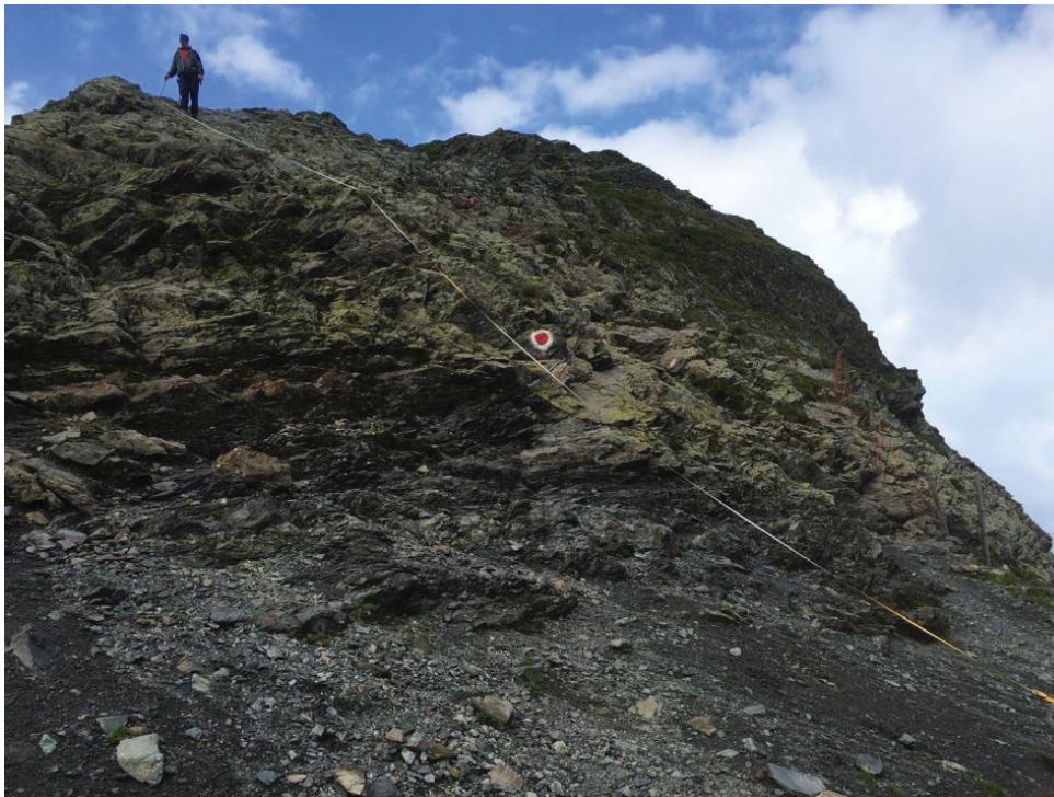
Figure 46: Eastern ridge of the Weinbichl. In the lower part of the picture are strongly sheared graphitic schists followed by gneisses, amphibolites and mica schists. The yellow line marks the measuring tape for the detailed profile shown in Figure 47 . The hiking path follows the ridge uphill. The person on the picture is 1.9 m tall.
