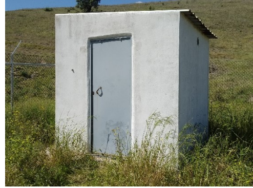
Figure 31 - Structure H: primary ventilation fan ancillary facility.
