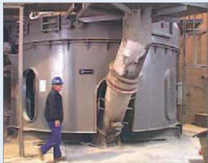
HOTDISC reactor after installation in Norway (6.0m diameter x 2.5m height)
